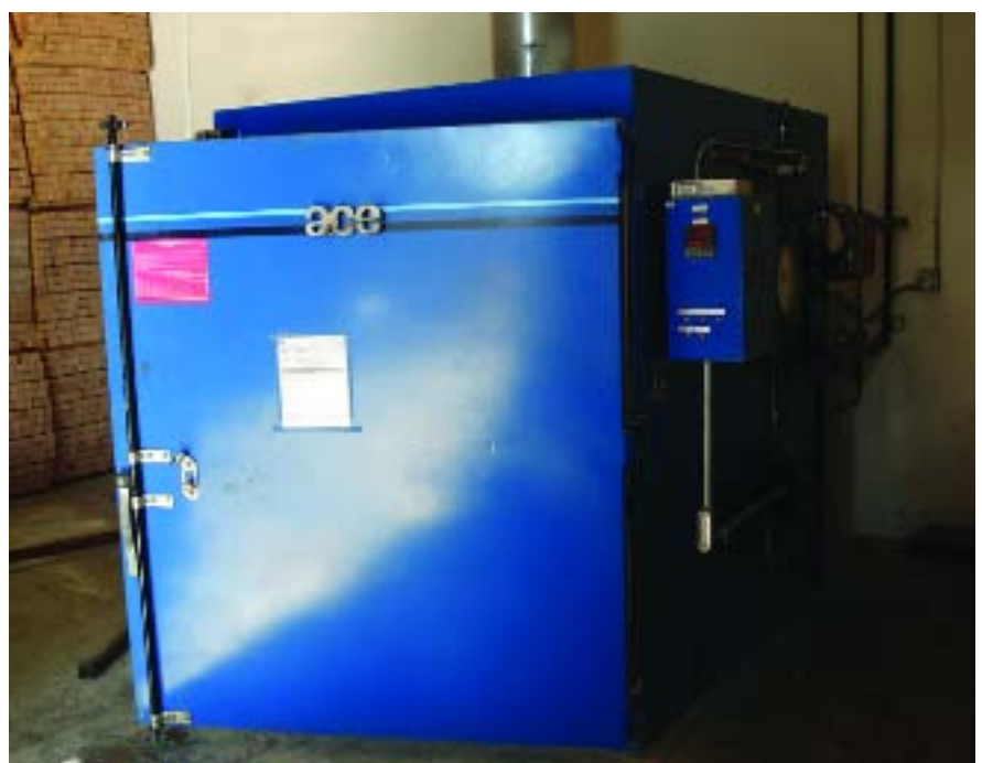
Hannibal Industries uses this burn-off oven to remove powder buildup from its hangers.
